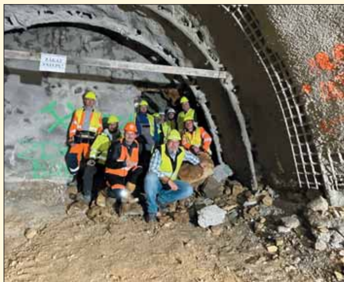
Obr. 8 První prorážka tunelu mezi šachtami Š9 a Š8 z 8. 10. 2025 Fig. 8 The first breakthrough of the tunnel between shafts Š9 and Š8 from 8/10/2025
