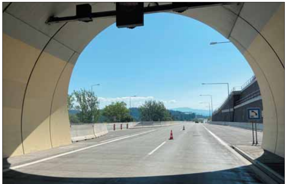
Obr. 2 Tunel Šibenik s CB krytom vozovky Fig. 2 Šibenik tunnel with cement concrete pavement
