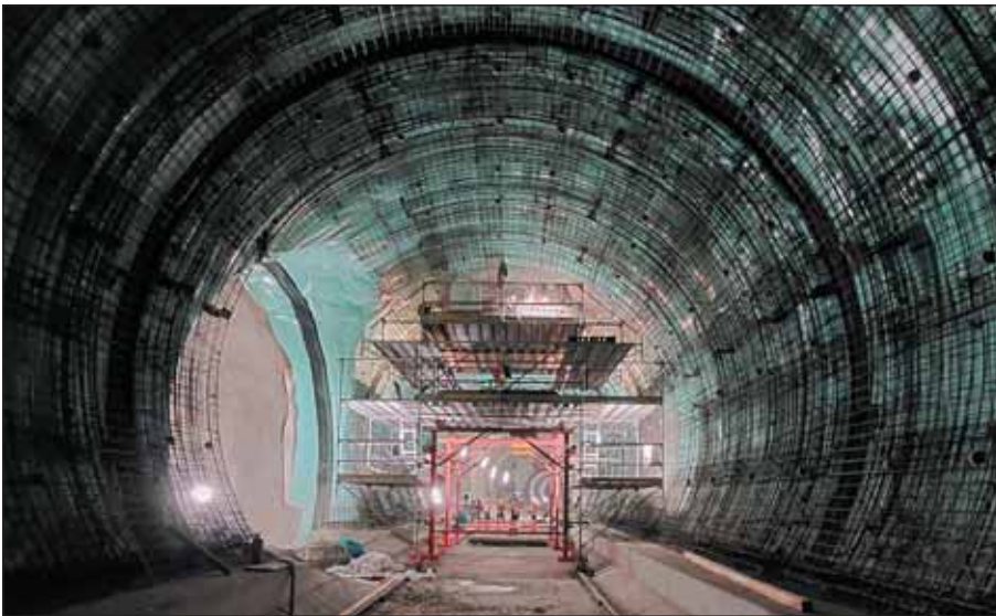
Obr. 5 Hydroizolace a armatura staničního tunelu Fig. 5 Waterproofing and reinforcement of the station tunnel
