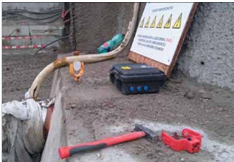
Obr. 3 Osadenie seismografu BRS 56 na portáli Fig. 3 Installation of the BRS 56 seismograph on the portal
