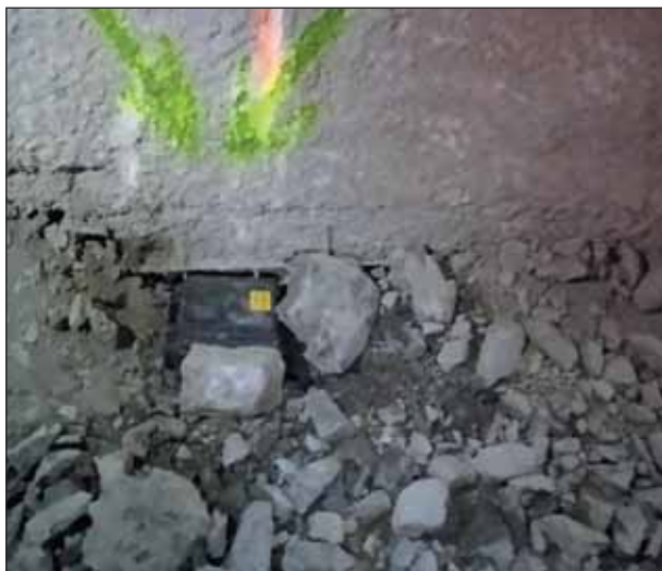
Obr. 2 Osadenie seismografu BRS 14 v tuneli Fig. 2 Installation of the BRS 14 seismograph in the tunnel
