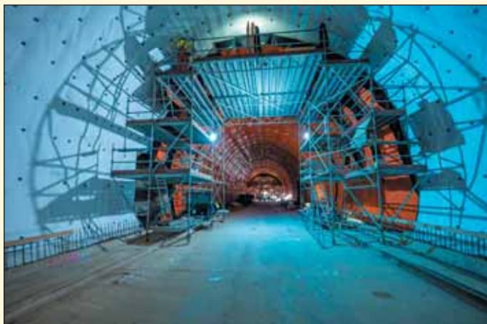
Obr. 1 Realizace izolace jižního tunelu Fig. 1 Installation of waterproofing in the southern tunnel tube
