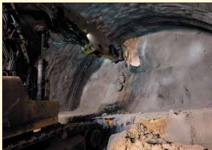
Obr. 2 Okamžik strojní prorážky severního tubusu tunelu Fig. 2 Moment of mechanical breakthrough of the northern tube of the tunnel
