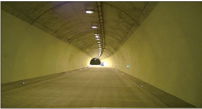
Obr. 7 Osvetlenie tunela v núdzovom stave Fig. 7 Tunnel illumination in the emergency state
