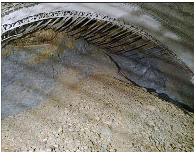
Obr. 1 Vysypávanie zeminy medzi ihlami v klenbe kaloty Fig. 1 Spilling of soil between needles in the top heading vault
