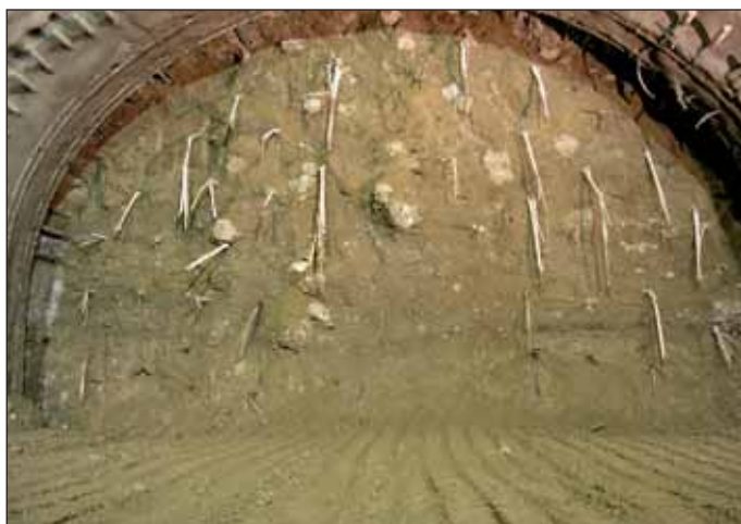
Obr. 2 Zajištění stability čelby dle metody ADECO-RS Fig. 2 Stabilisation of the face according to ADECO-RS principles
