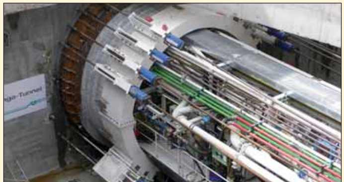
Obr. 5 Pohled na zarážku štítu v Hafens City v Hamburku Fig. 5 A view of the tunnel opening work for the TBM excavation of the HafensCity tunnel in Hamburg
