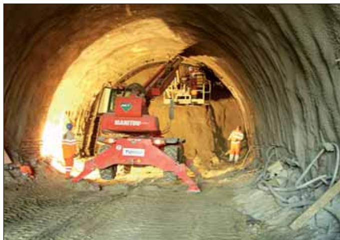
Obr. 5 Vystužovanie ostenia tunela sieťovinou Fig. 5 Reinforcing of the tunnel lining with steel mesh
