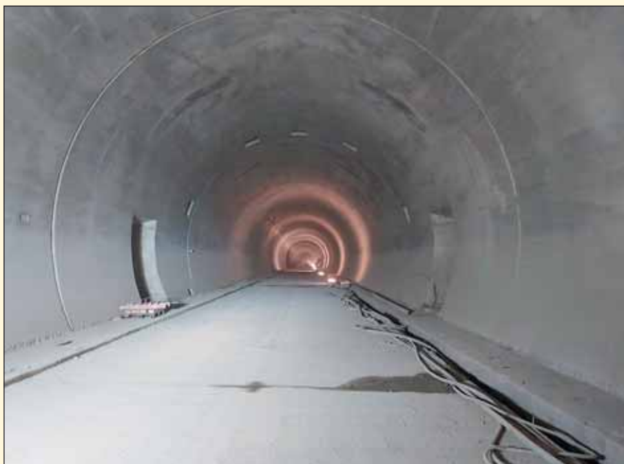
Obr. 7 Južná tunelová rúra pripravená na budovanie chodníkov Fig. 7 Southern tunnel tube prepared for carrying out walkways
