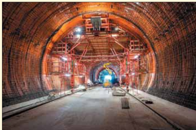
Obr. 2 Realizace armatury jižního tunelu Fig. 2 Placement of reinforcement in the southern tunnel tube
