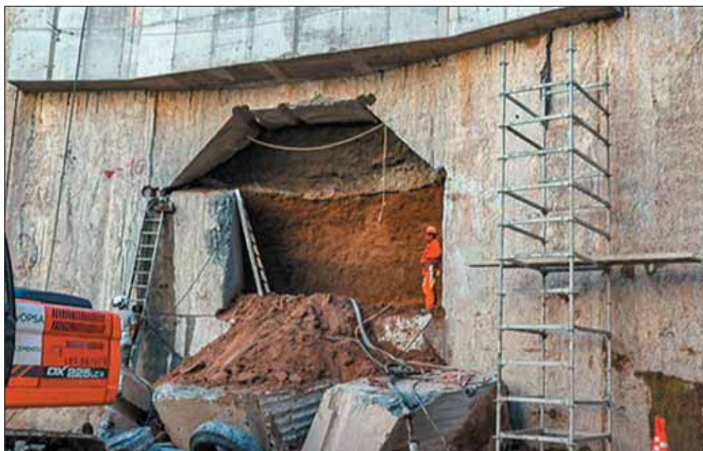
Obr. 6 Záber z otvárania steny šachty Fig. 6 Snapshot from opening of a shaft wall
