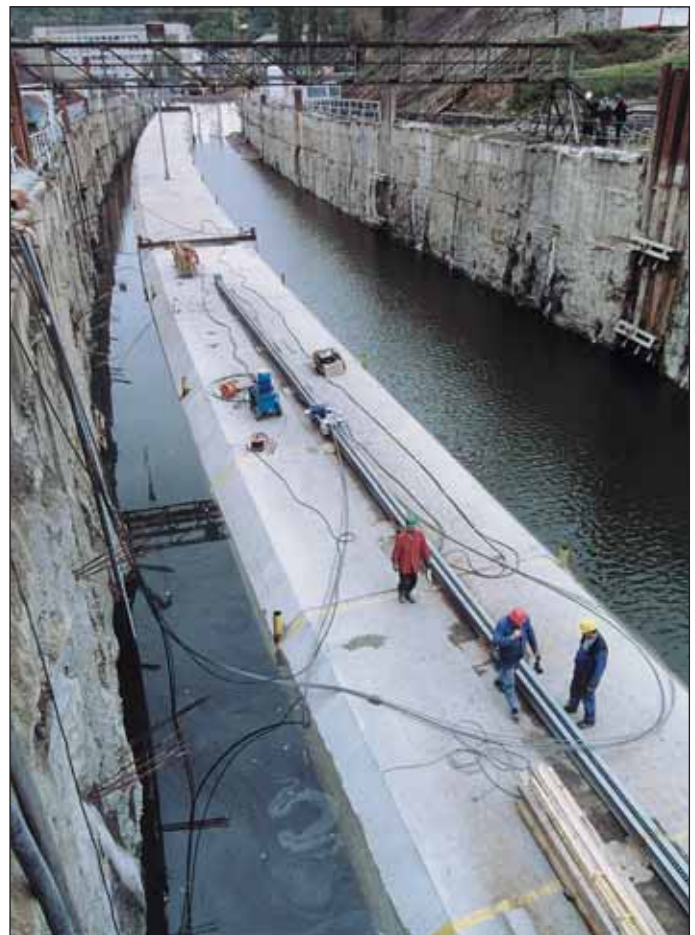
Obr. 7 Tubus traťového tunelu v zaplaveném doku Fig. 7 Tube of running tunnel in flooded dock
