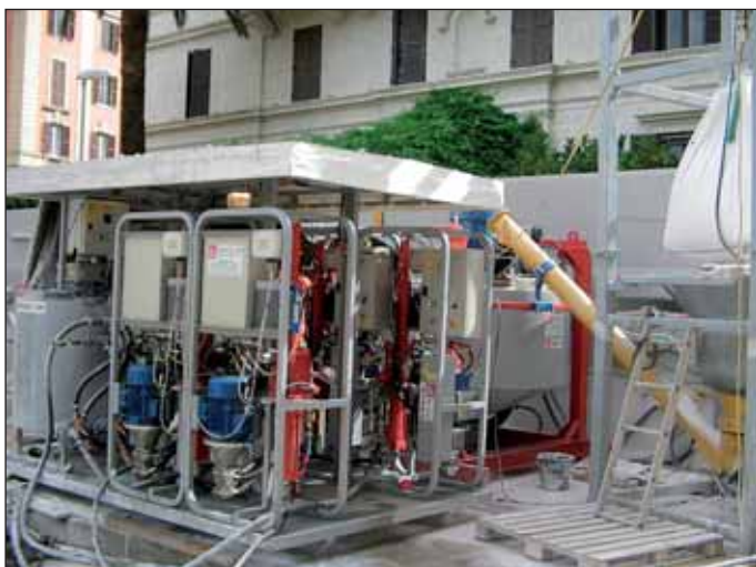
Obr. 7 Zmiešavacie zariadenie Fig. 7 Mixture central station
