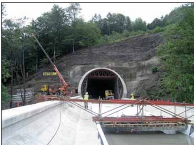
Obr. 6 Tunel Malá Huba (v provozu od r. 2005) Fig. 6 Malá Huba tunnel (in operation from 2005)
