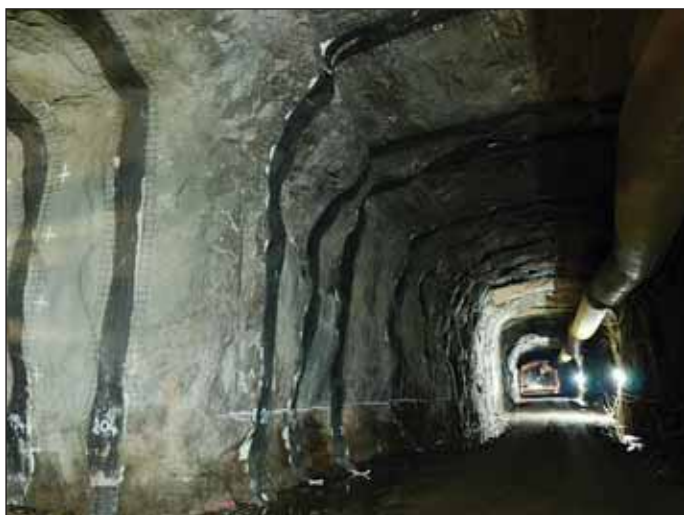
Obr. 11 Systematicky instalované organizované svody Fig. 11 Systematically installed elements of the organised water collection system
