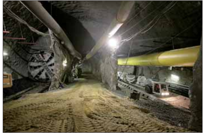
Obr. 12 Stanice Petřiny, provizorní segmenty pro S-609 Tonda; S-610 Adéla ve stanici Fig. 12 Petřiny Station, temporary segments for S-609 Tonda; S-610 Adéla in the station
