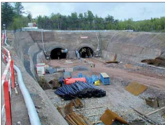
Obr. 11 Tunel Panenská (v provozu od r. 2006) Fig. 11 Panenská tunnel (in operation from 2006)
