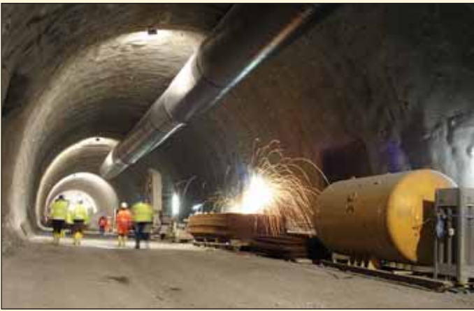
Obr. 3 Upravená počva v úseku s bobtnavými horninami Fig. 3 Modified invert in the section passing through swelling ground
