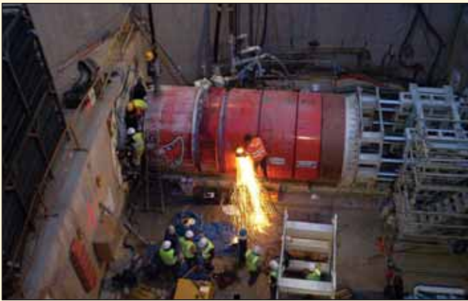
Obr. 1 Pohled do šachty s mikrotunelovacím strojem ISEKI Unclemole CTP Fig. 1 View down the shaft with ISEKI Unclemole CTP microtunnelling machine
