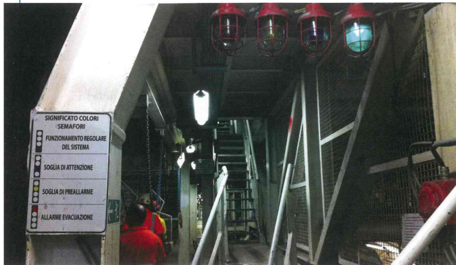
Above: Methane warning system at the lowest alert level, for normal running
